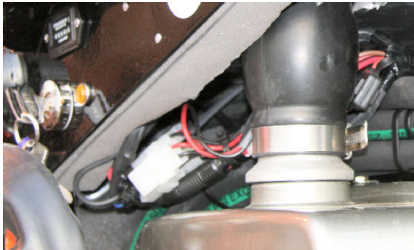
Fig 5-29 Engine cable loom 6
