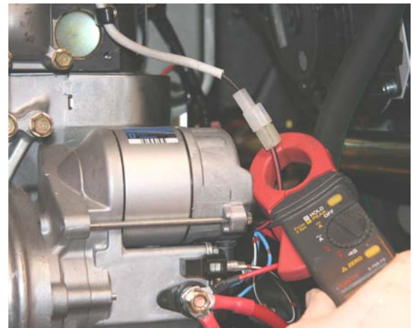
Fig 4-3 Clamp meter current check
