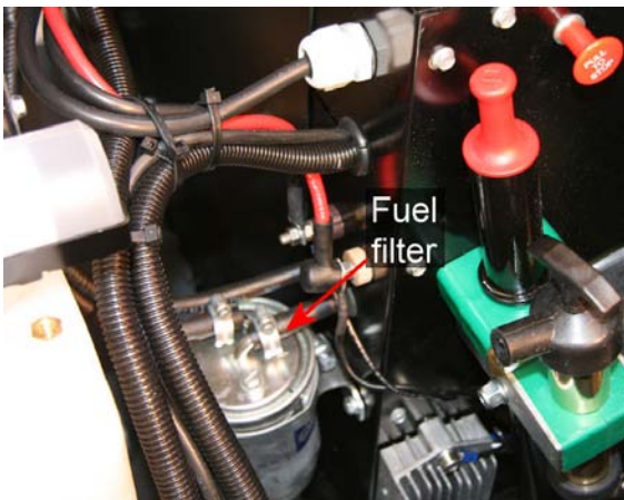
Fig 3-13 Fixed fuel filter
