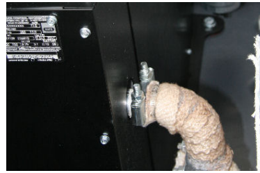
Fig 5-13 Engine exhaust outlet
